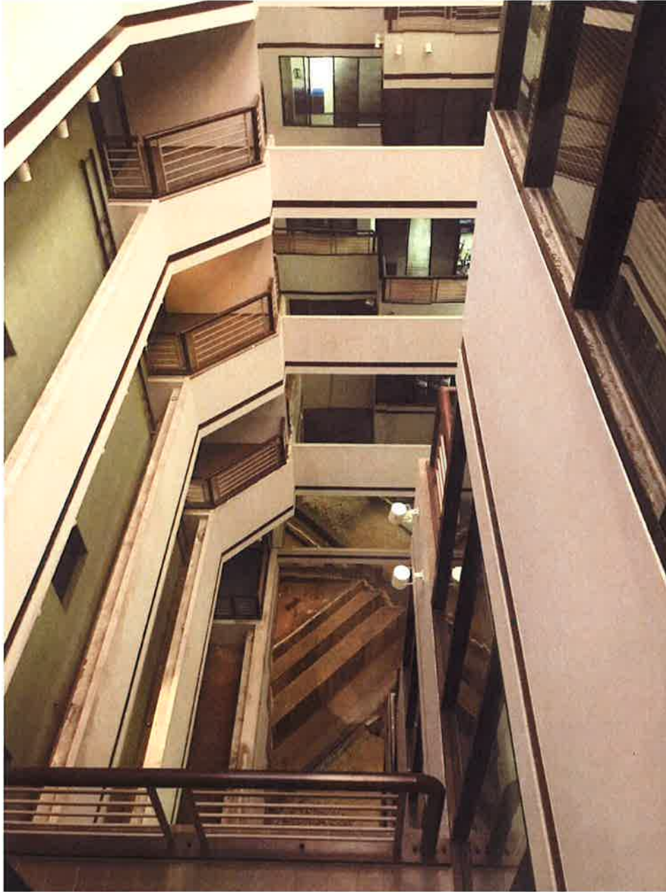
Above: Deteriorated atrium interior balconies.
