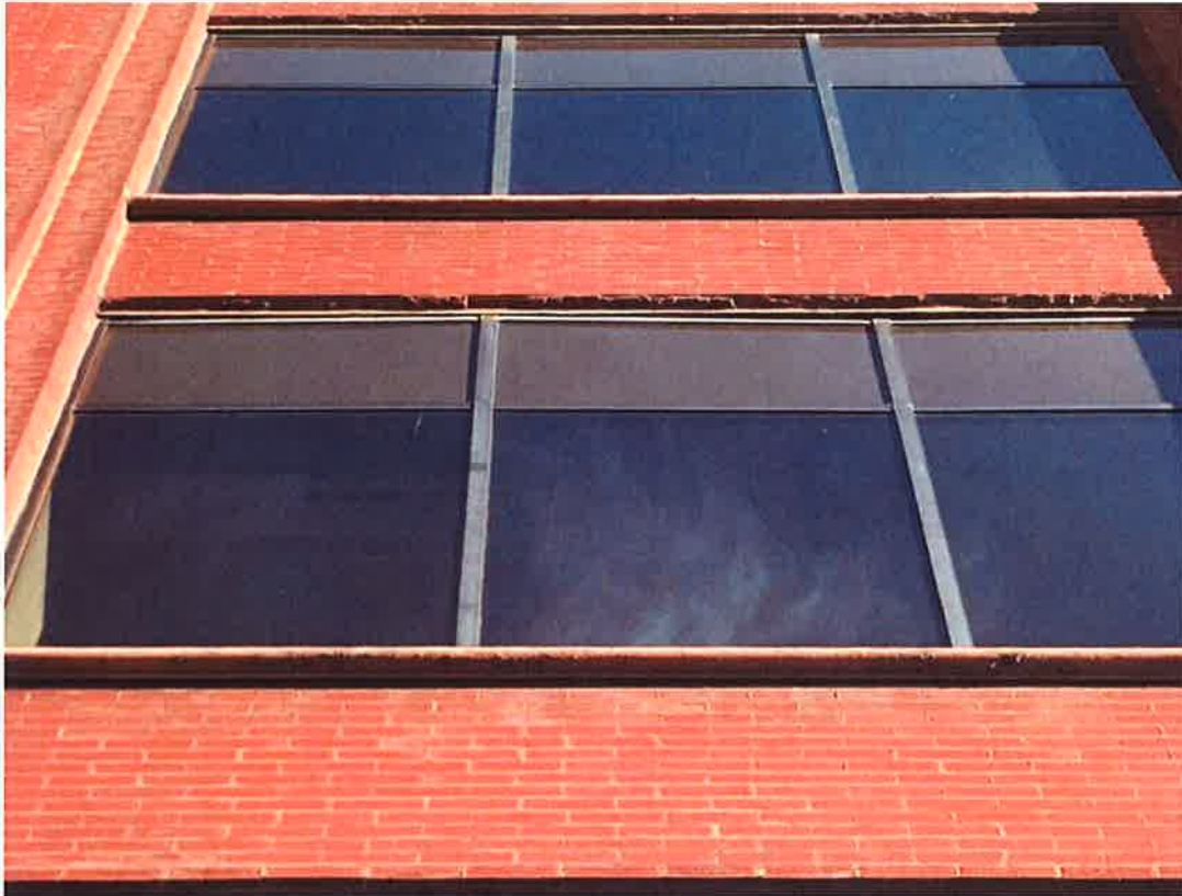
Above: Deteriorated window sill and lintel.
