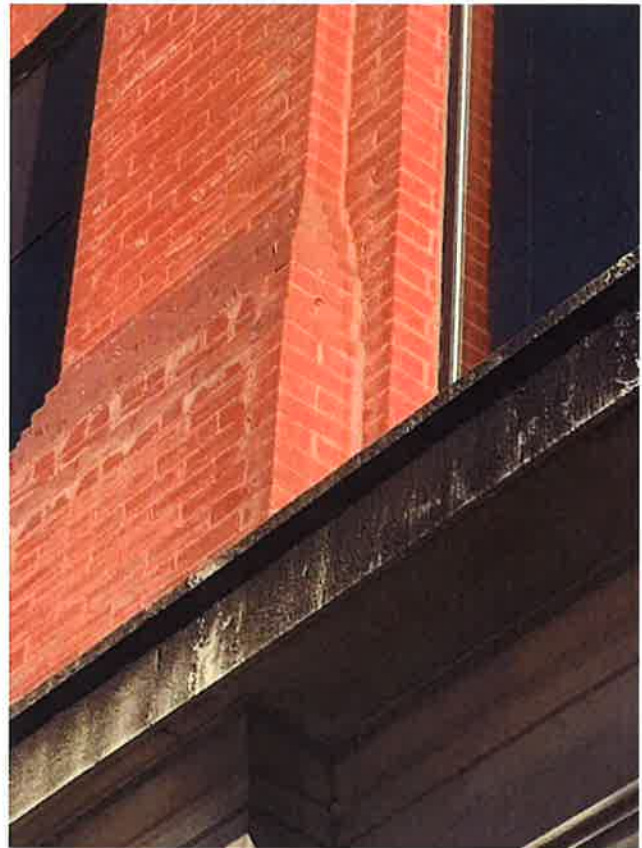
Above: Deteriorated bricks and mortar.
