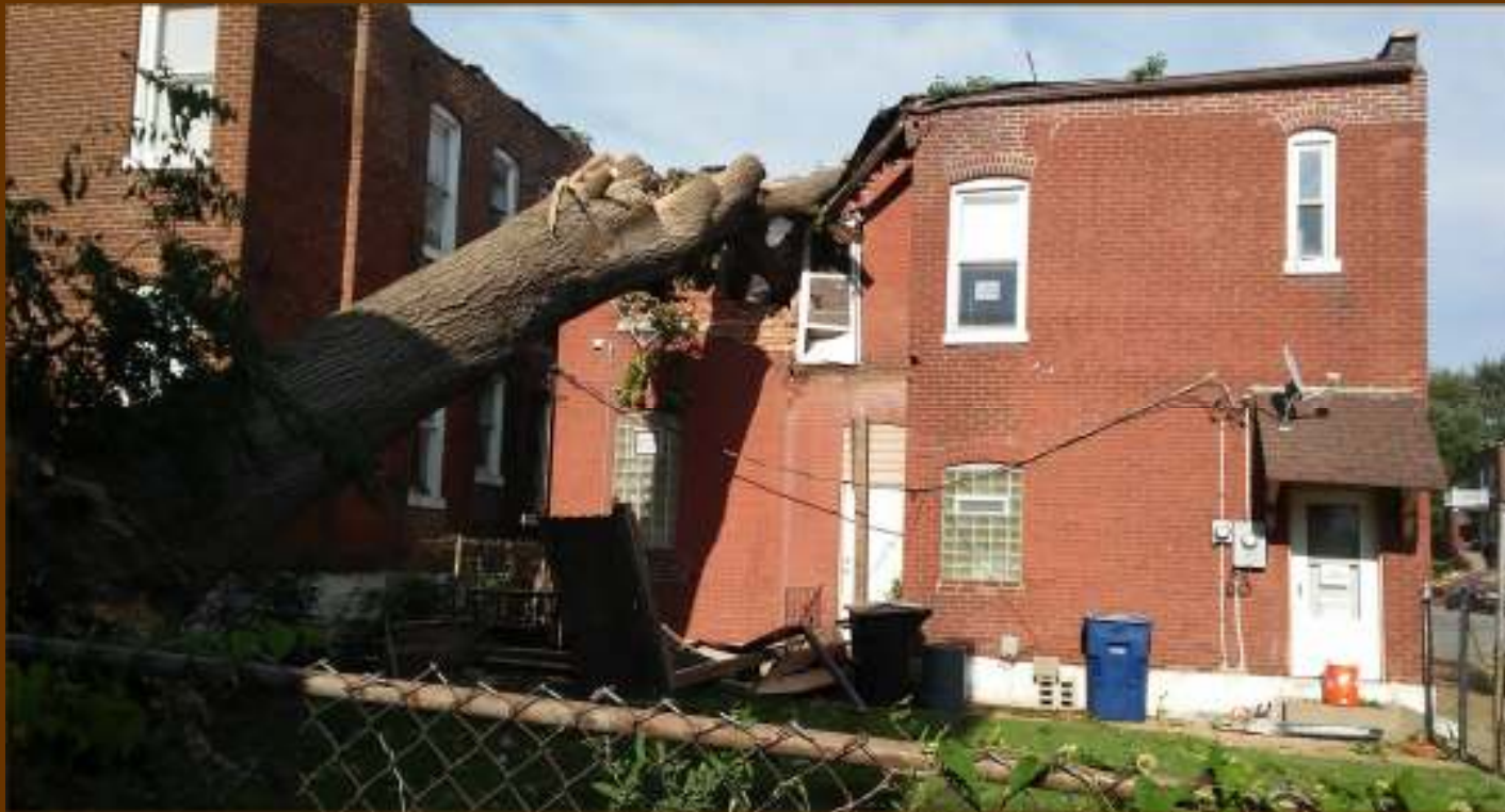
PHOTO OF BUILDING WITH FALLEN TREE
