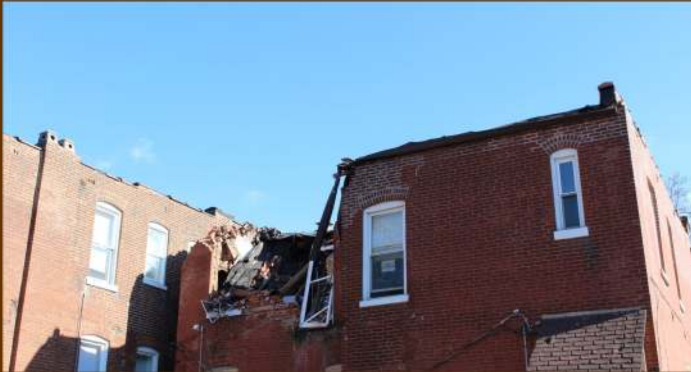
CLOSE-UP OF DAMAGE
