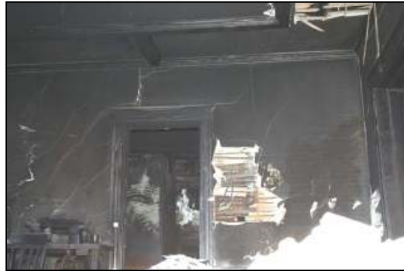
Interior room visible through collapsed area
