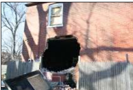
Area of collapse in east wide wall
