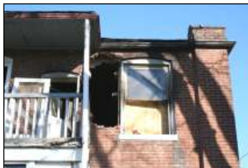
Loss of brick in rear elevation
