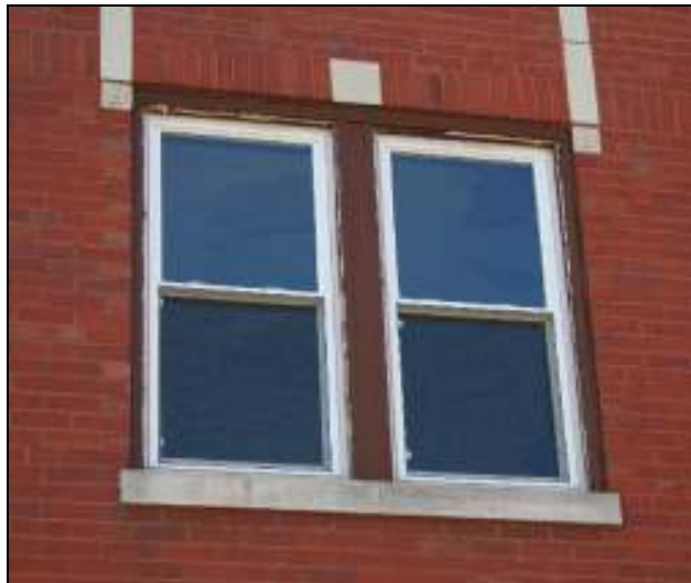
VINYL FRONT WINDOWS INSTALLED WITHOUT A PERMIT
