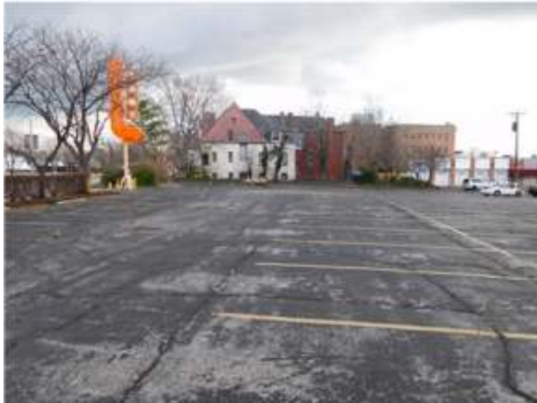
Cracks in surface parking lot, 3514-20 Dr. Samuel T. Shepard Dr.
