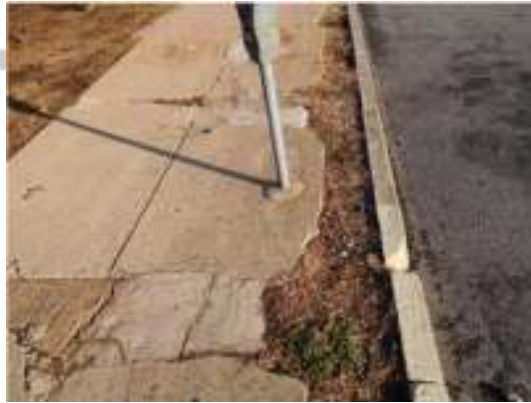
Cracked sidewalk, 3517-25 Washington Blvd.
