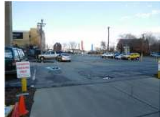
Surface parking lot with potholes, 3517-25 Washington Blvd.
