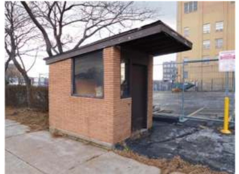
Deteriorated structure, 634 N. Grand Blvd.
