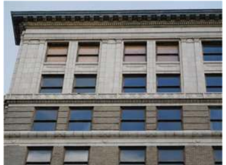
Boarded-up windows, 634 N. Grand Blvd.
