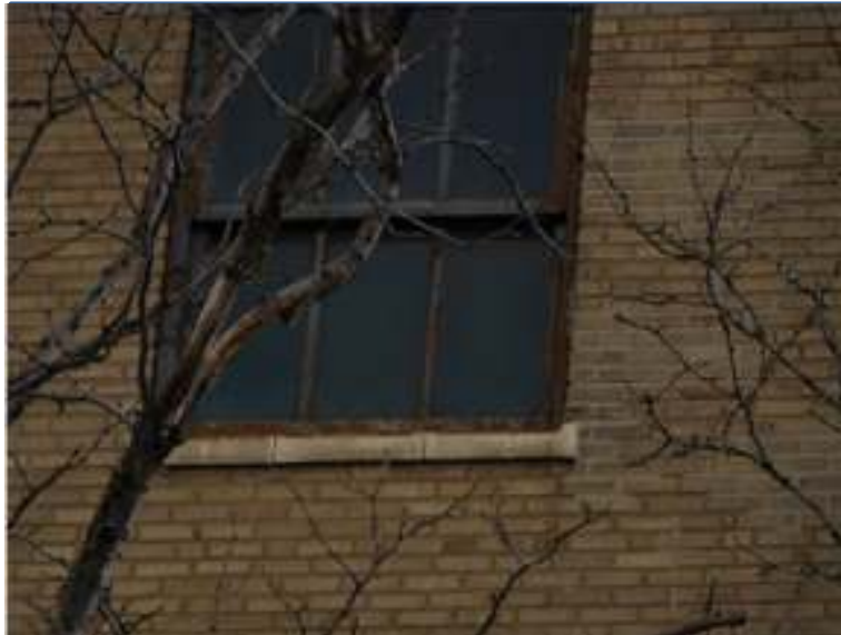
Rusty window frame, 634 N. Grand Blvd.
