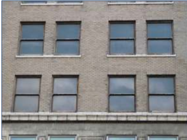
Deteriorated windows/dirty terra cotta, 634 N. Grand Blvd.
