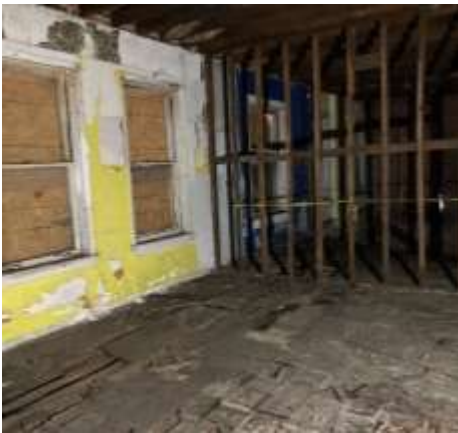
As the photo on the right shows, the building has been structurally stabilized but some of the interior floors still require re-building.
