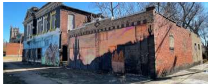
A second building (shown above), with 1904 sq.ft., comes with the parcel but was not stabilized and has a completely collapsed interior.
